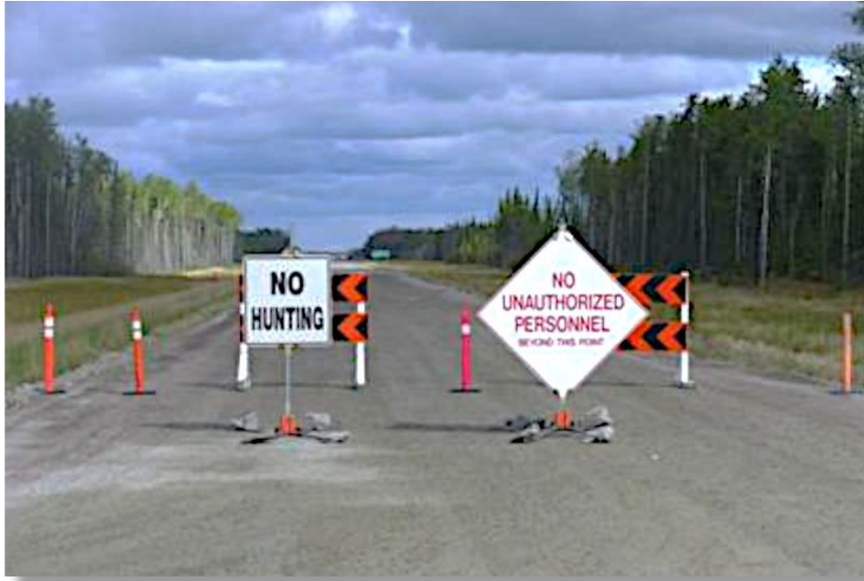
Photograph 9-23: Barricades and Signage Installed in the P1-All-Season Road Corridor During the Construction Phase to Discourage hunters
